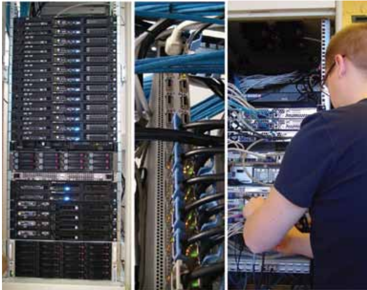
Cloud computing - physical infrastructure: servers, storage, Infinband switch
