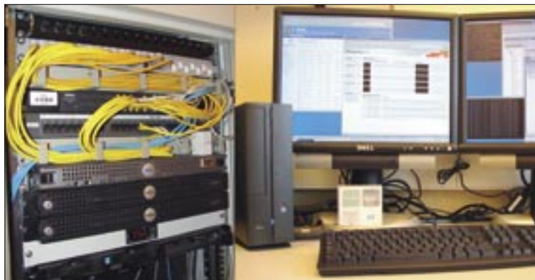
Communication infrastructure within the Laboratory
